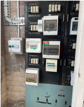
NS1: Switch board backing. Auxiliary power boards.
