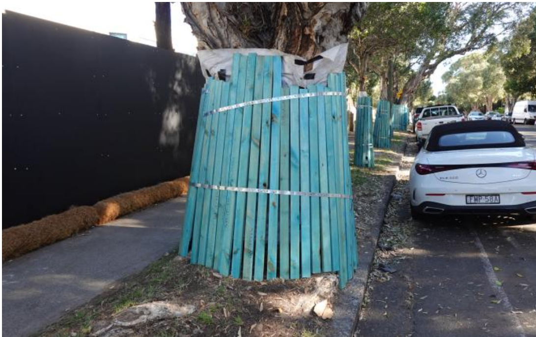
Figure 3.3 – Acceptable Trunk Protection batten installation – height of boards to be at least 2.4m or to the first branches. (Photo: Arterra)
