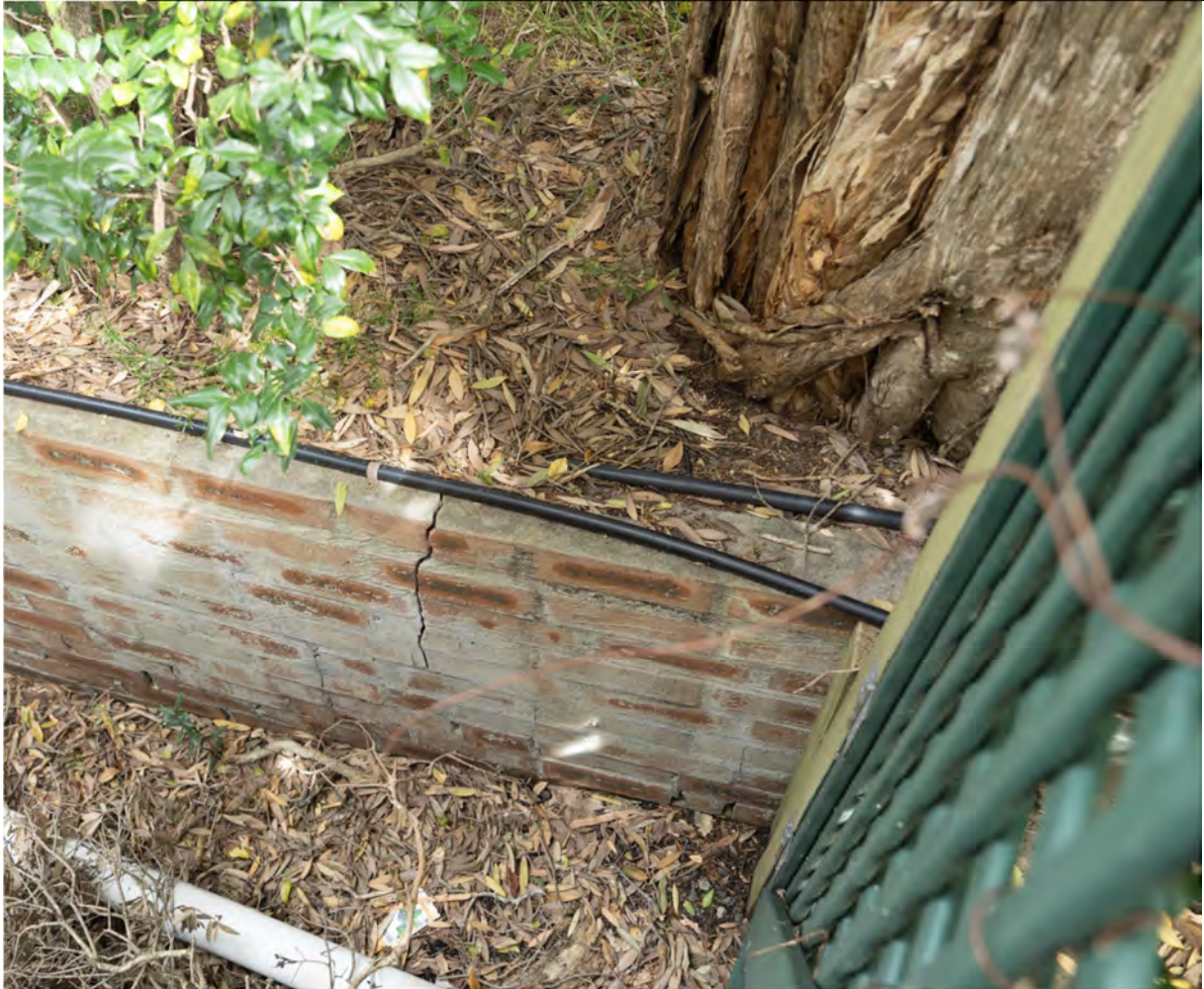
Image 5: Failure of a boundary masonry wall adjacent to PT16.
