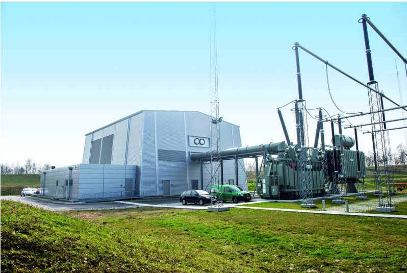
Figure 3 Example of Synchronous Condenser
