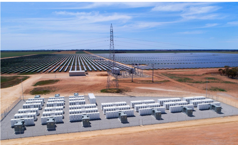
Figure 4 Example of Batter Energy Storage System
