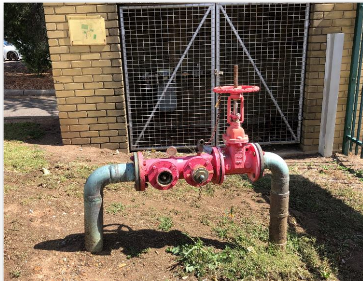
Figure 12: Fire Brigade Booster Assembly
