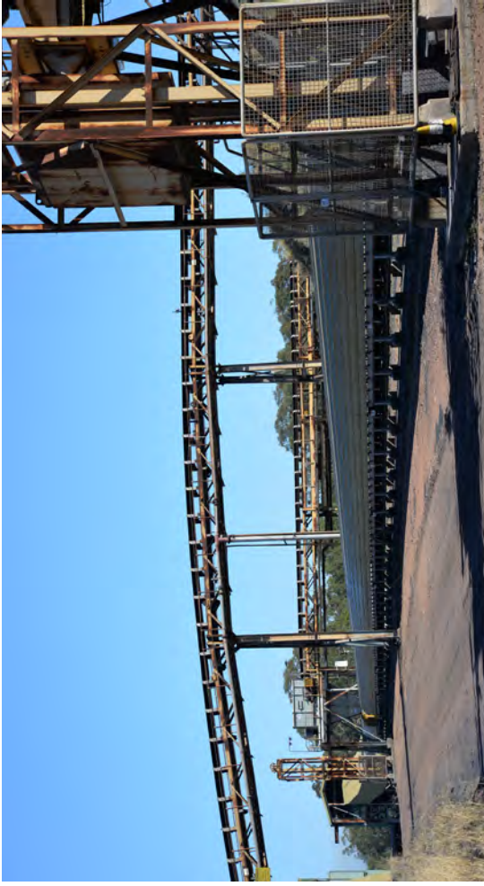
Existing coal processing and loading equipment.
