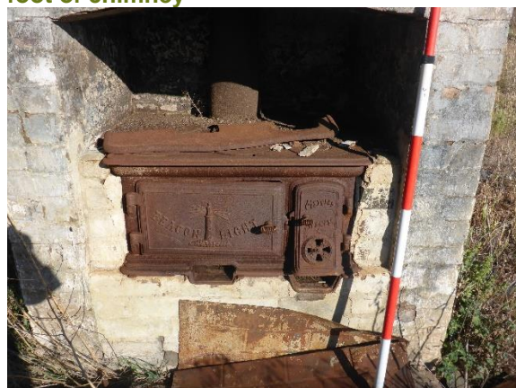
Figure 30: Brick chimney containing Metters Sydney stove. Pressed metal ceiling material at foot of chimney
