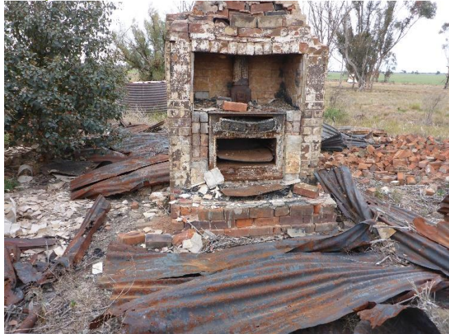
Figure 18: Closer view of chimney, view north complex (Photographed by M Lever, 12 October 2018)
