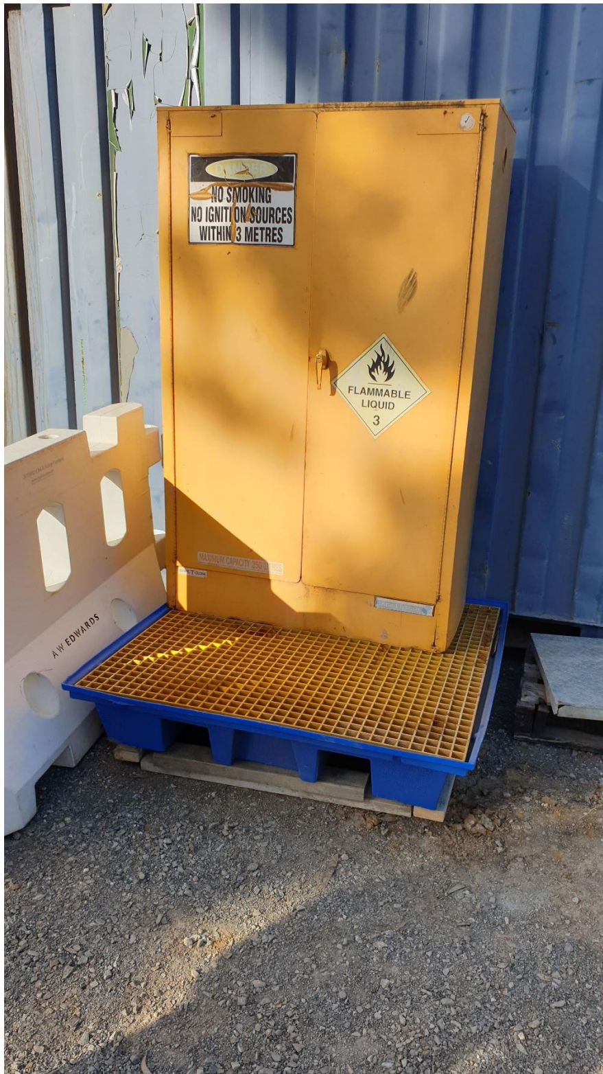
Plate 5 – Flammable liquid store on spill pallet
