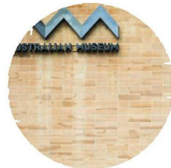
EXTERIOR SANDSTONE CLADDING LOCATION: FACING TO PARKES FARMERS WING DESIGN INTENT: TO MATCH THE EXISTING HERITAGE FACADE
