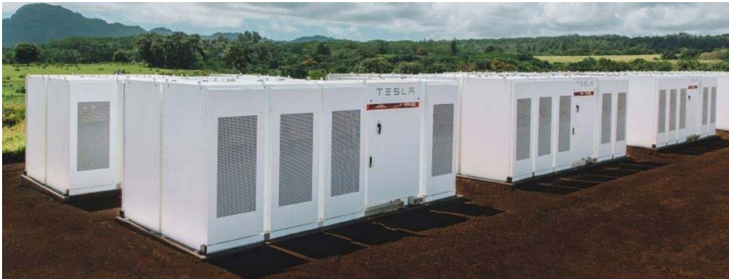
Figure 2-4 Example Battery Storage
