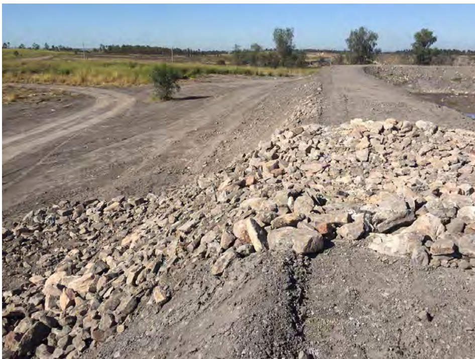
Photo 2 Rock lined overflow section on the eastern wall of the detention basin
