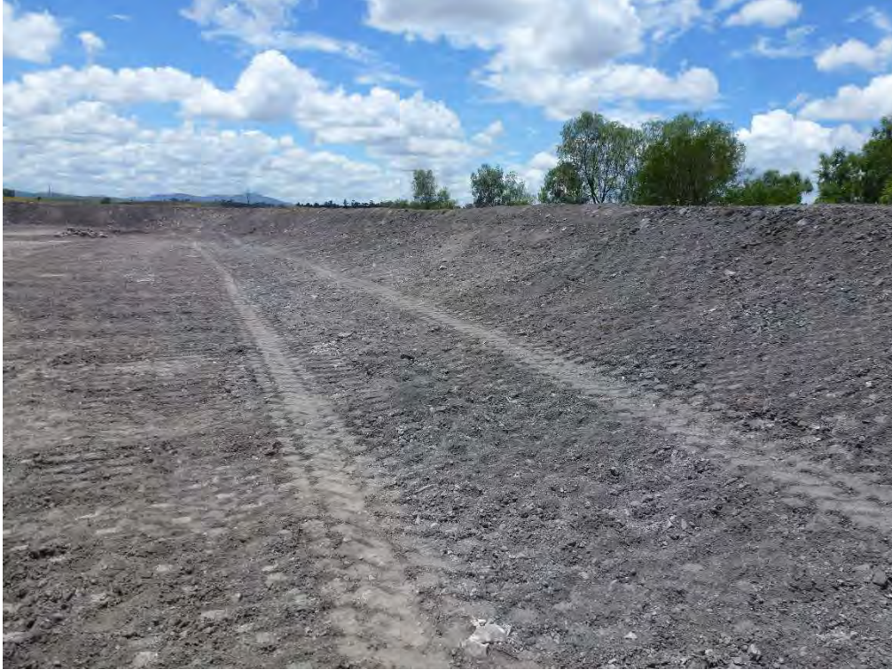
Photo 3 Looking east along the upstream face of the southern sedimentation basin embankment
