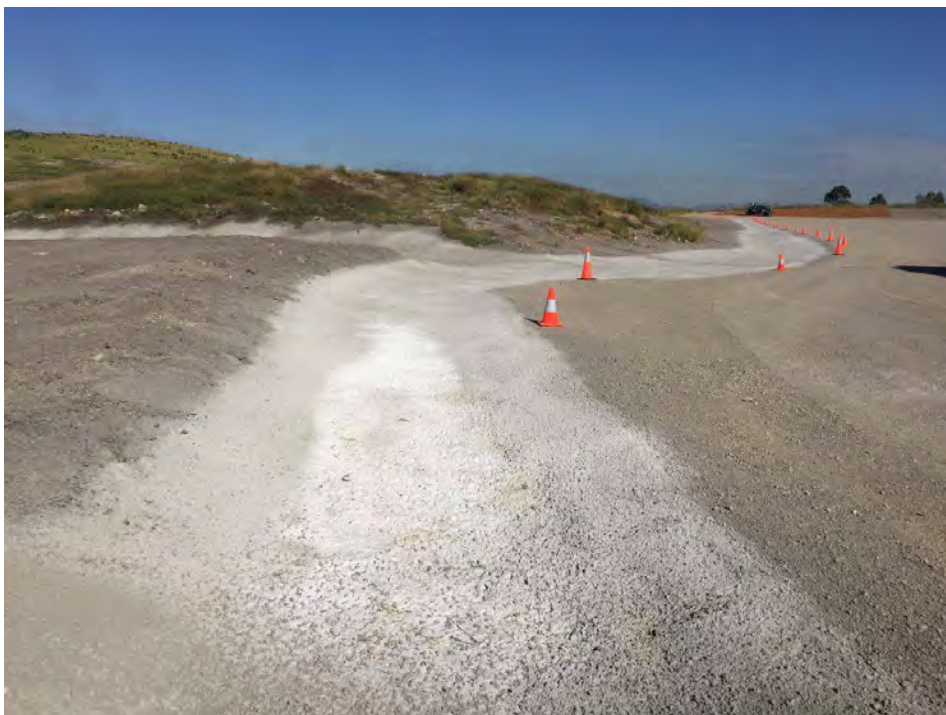
Photo 6 Looking along the composting pad southern perimeter surface drain, leading to the spillway
