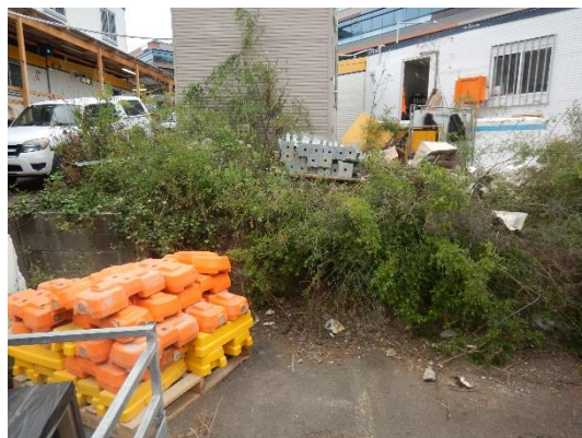
Figure 6.8: Retaining wall located at the south of the property (facing west) (Photographed by R. Taddeucci, 24 September 2018)
