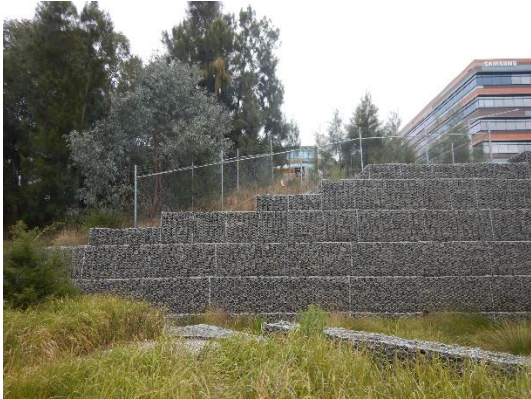
Figure 4.13: View west of retaining from outside the property (Photographed by R. Taddeucci, 24 September 2018)
