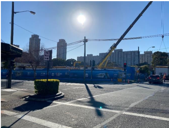
Picture 1 South western corner of site, located at the corner Wellington Street and Botany Road
