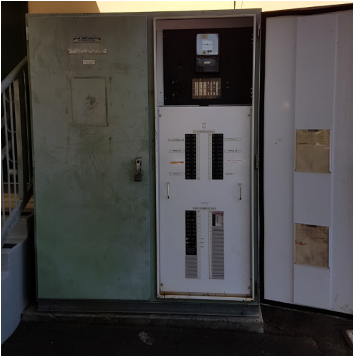
Figure 3 – Existing School Main Switchboard
