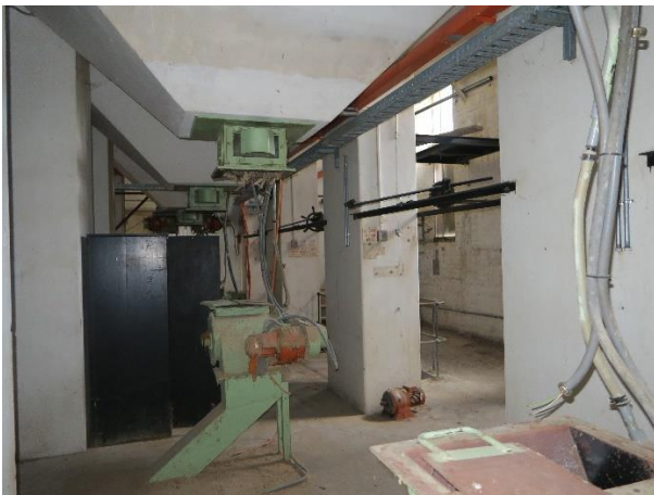
Figure 14 – Malt Silos 1, 2, 3, 4, 5, 6, 7 and 8 (metal equipment and base of reinforced concrete silos) (all) in building 23 (ground floor/ level 1).
