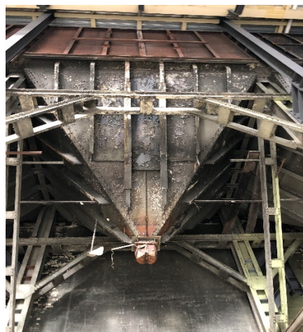
Figure 17 – Detail of one of three coal hoppers
