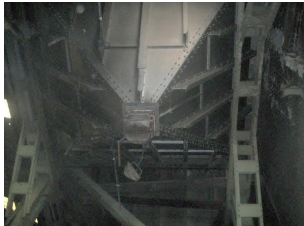
Figure 17 – One of the three coal hoppers within Building 30.
