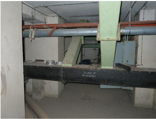
Figure 16 – The basement conveyor and associated plant, part of which is to be retained and displayed via the viewing panel in the ground floor
