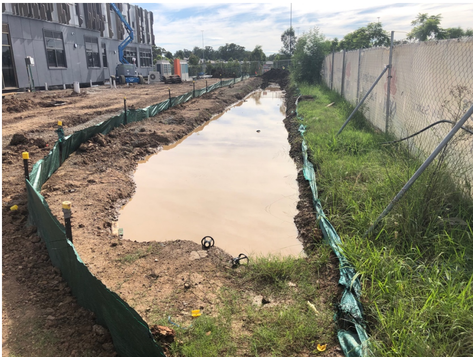
Figure 14 Boundary sediment controls - collapsed sediment curtain
