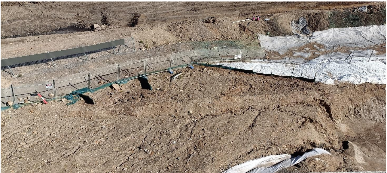
Photograph 6 – NICB interface - Basin 2
