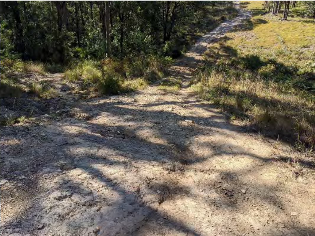
Plate 6.9 Example of erosion and topsoil disturbance as a result of ongoing track use on the slope in SU5
