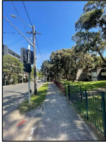
Figure 100: SU4 – Concrete footpaths and front yards of social housing, view west along McEvoy Street showing declining slope
