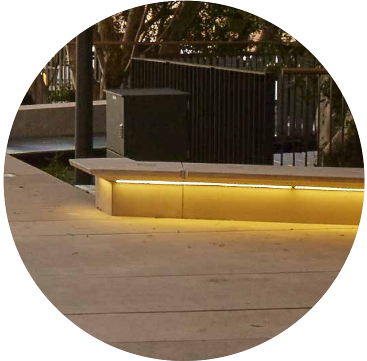
Strip Lighting Recessed, under bench light
