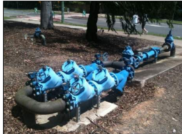
Figure 11 Culloden Road Main Meter
