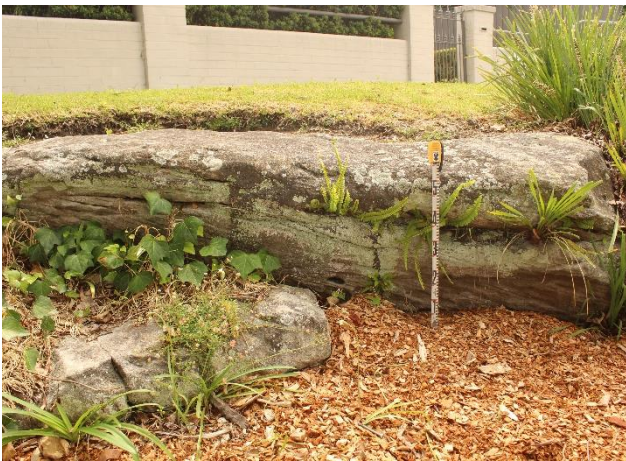
Figure 27 - View west of sandstone outcrops in the vicinity of the subject area's eastern edge.
