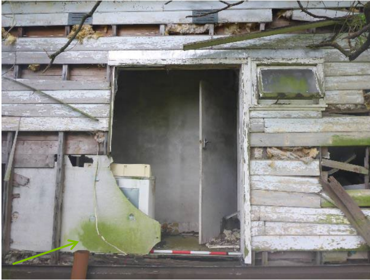
Photo 14 Exterior view of residential building [2] showing holes in walls, fibro cladding and asbestos (as indicated by orange arrow)
