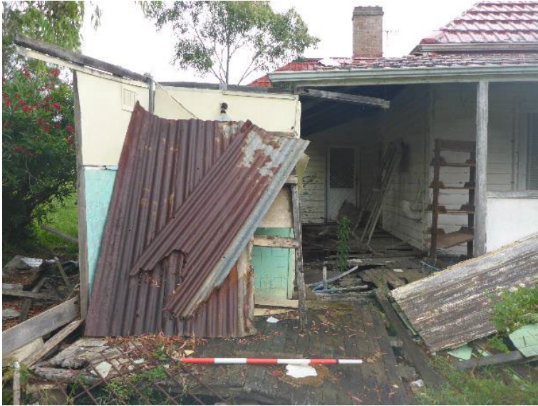
Photo 17 Exterior view of residential building [2] showing remains of tiled room, facing south
