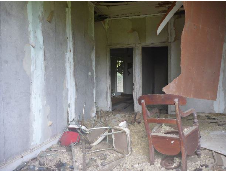
Photo 15 Interior view of residential building [2] showing condition and exposed insulation and asbestos
