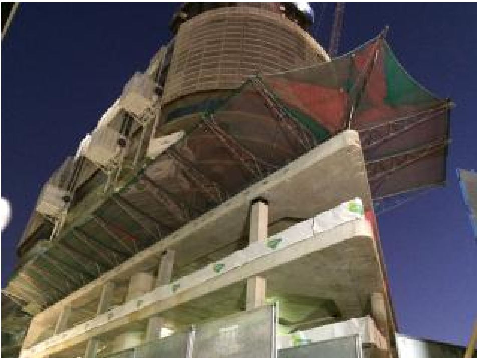
Figure 15 – Secondary Edge Protection - WorkRight Fan & Netting
