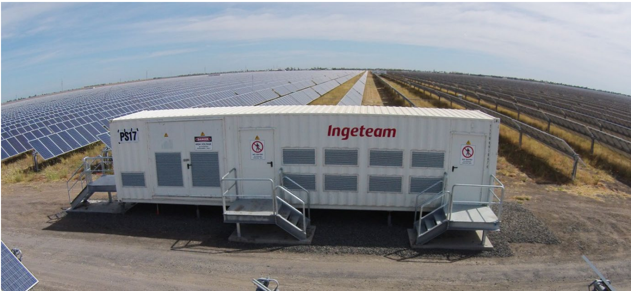
Photograph B.2 Containerised inverter solution with PV module rows
