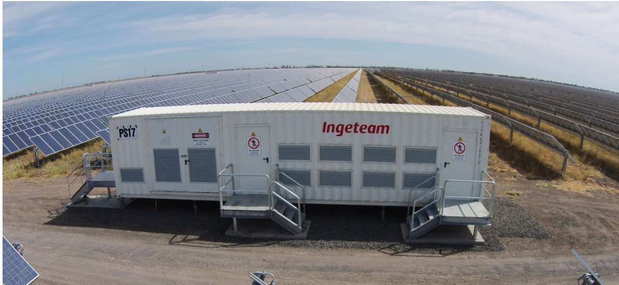
Photograph 4.2 Inverter surrounded by PV module rows (Source: Ingeteam 2018)
