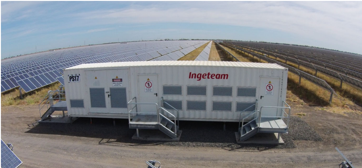
Photograph 2.2 Containerised inverter solution with PV module rows (Source: Ingeteam 2015)
