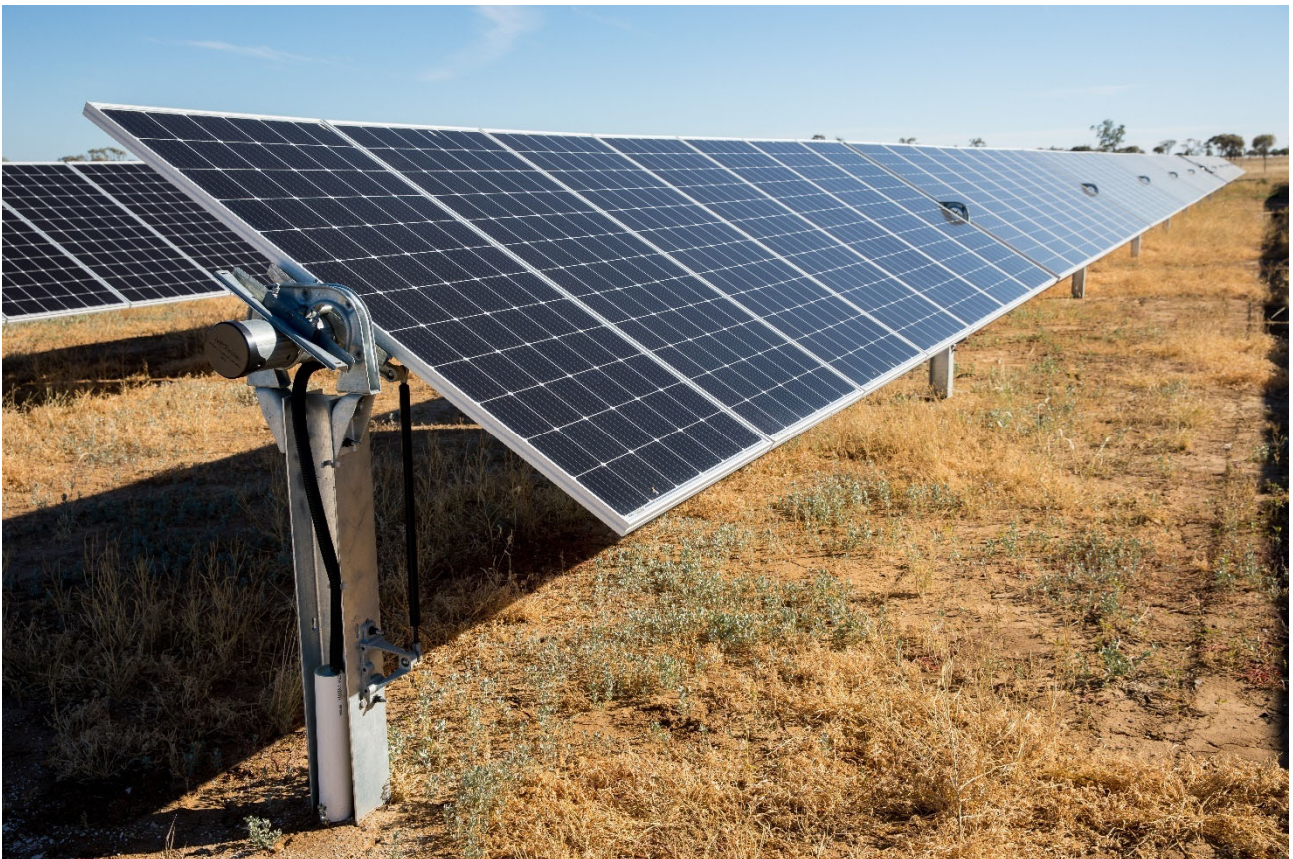
Photograph 2.1 PV module row with single axis tracking technology (Source: NexTracker 2018)
