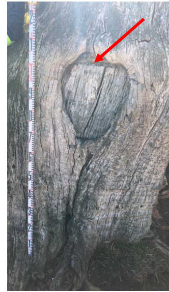
Plate 6.47 NE61 showing evidence of damage at the upper edge of the scar where overgrowth has receded, northern array area.
