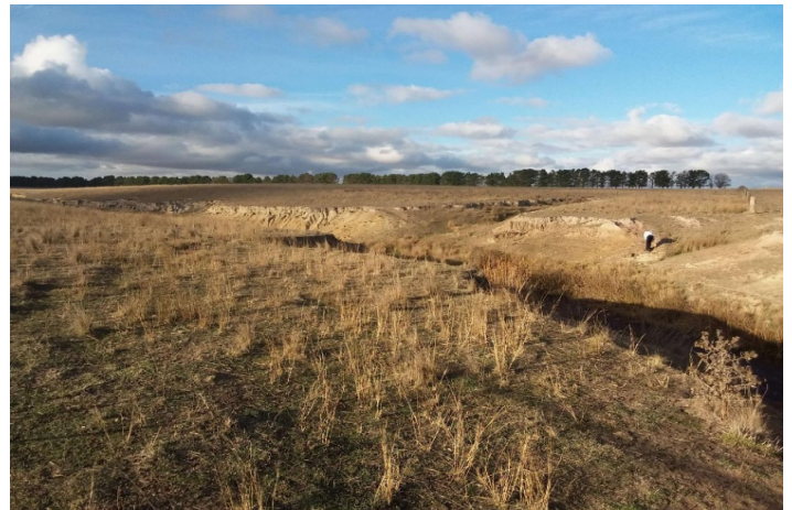
Plate 6.18 Unnamed 3 rd order watercourse showing deeply incised and eroded banks: T61, northern array, view north.
