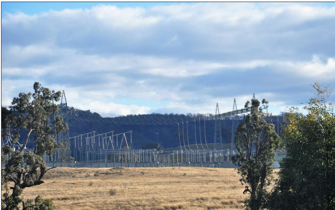
Figure A-7 Wollar 500/330kV substation.
