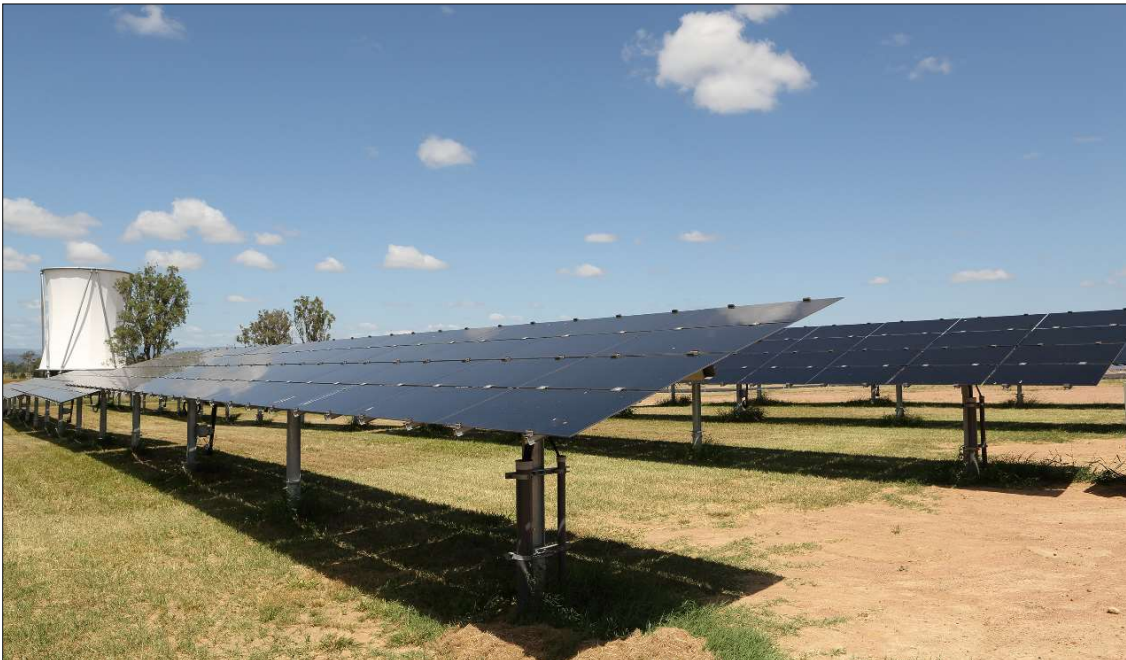
Figure A-4 Typical single-axis tracking system.
