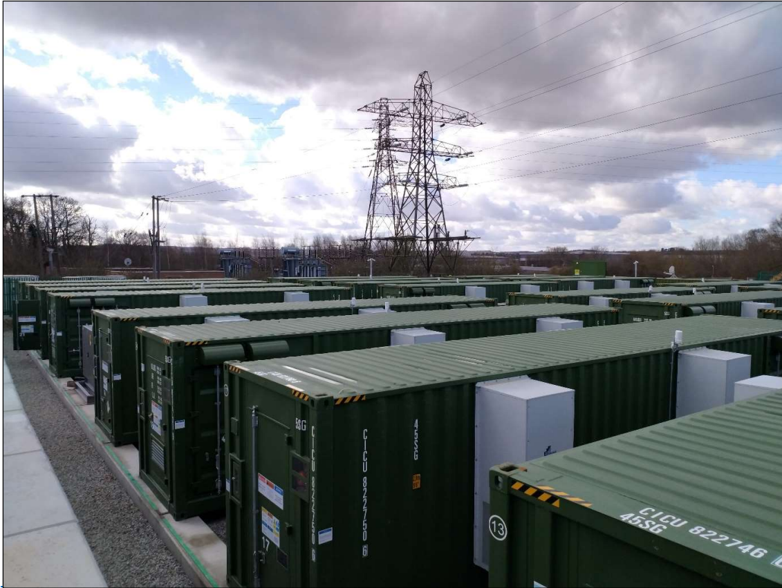
Figure A-12 Typical battery storage units, located together.
