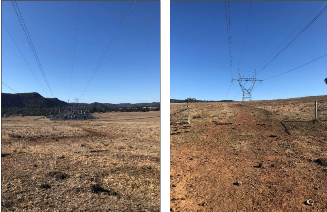
Figure A-8 330kV transmission line within 60m easement traversing the proposal site and connecting to the Wollar substation.
