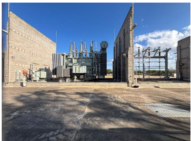
Figure 8 Existing transformer and vacant transformer bay
