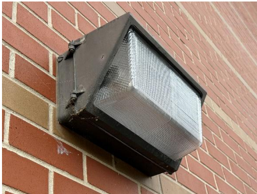
Figure 2 – Thorn Wallpack Luminaire Main Building Wall Light
