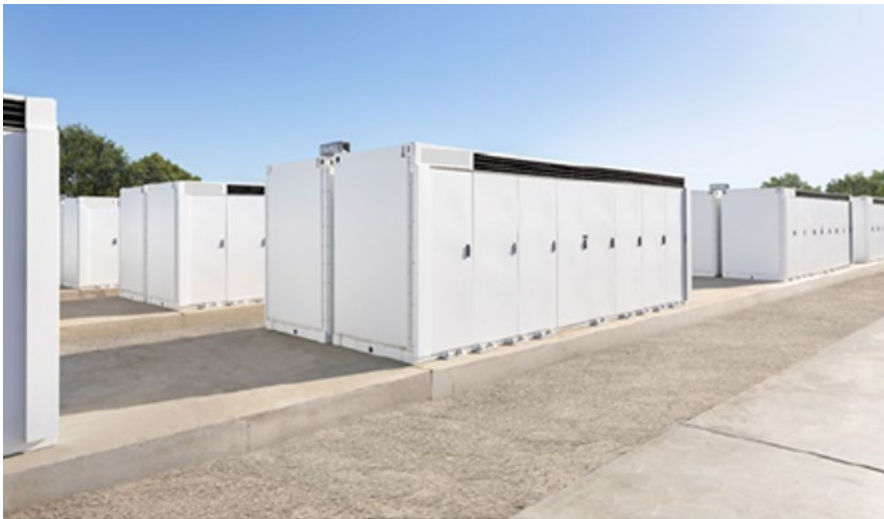
Figure 3-2: Typical BESS site
