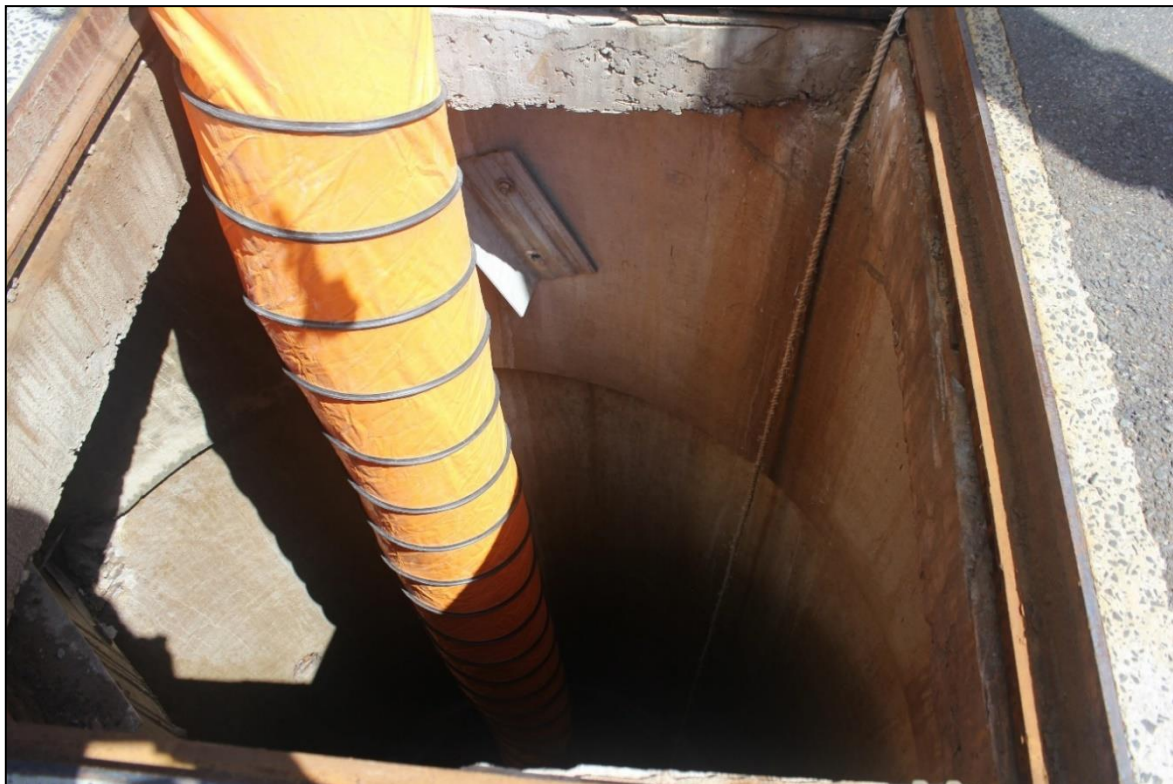
Figure 3.3: Cast concrete collar sitting on top of the original shaft masonry, looking west.
