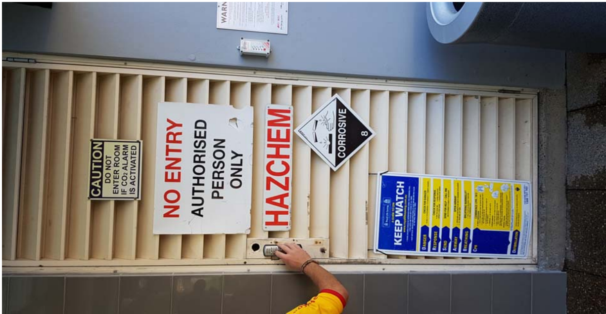
Photo 10 - Chemical storage room for pool to south-west of stadium
