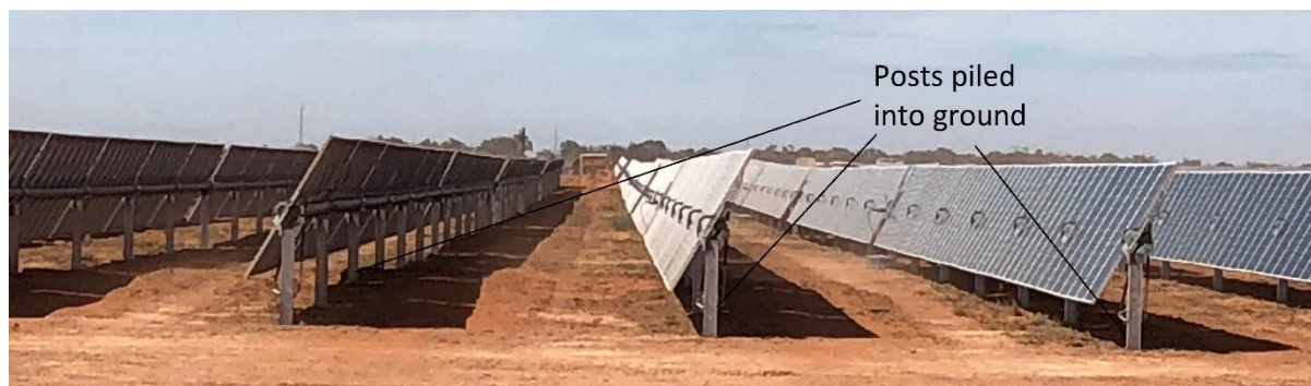
Figure 5 Posts Supporting the Tracking System
