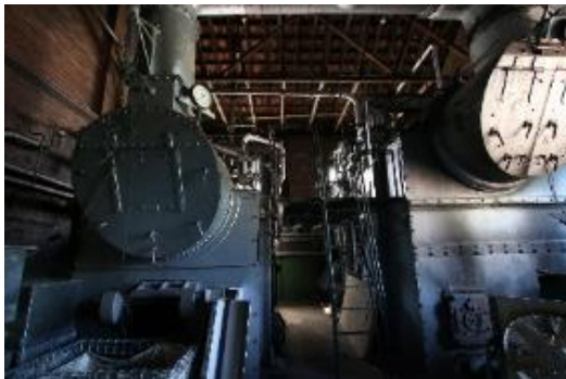
Plate 17 Steel coal fired boilers
