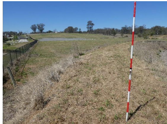
Plate 18. Facing east from the top of the rise of the dam. Carpark in midground.
