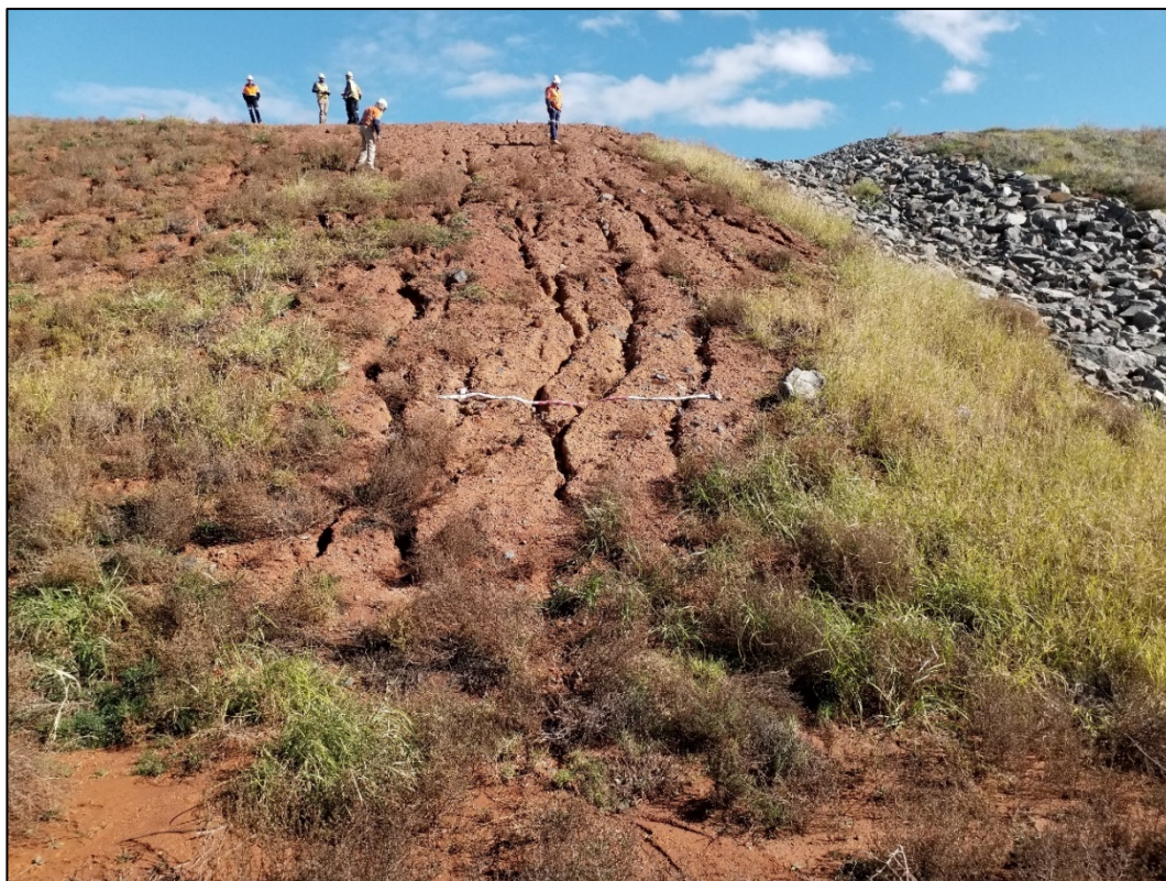
Photograph 6. Rill erosion observed on the batter of WRE #3. Likely related to disturbances associated with construction of the batter chute.
