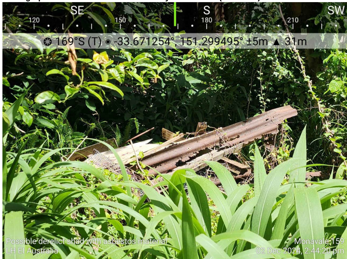
Photograph 2: Possible derelict shed at the southern portion of the site identified as a source of potential ACM (2/12/2024).
