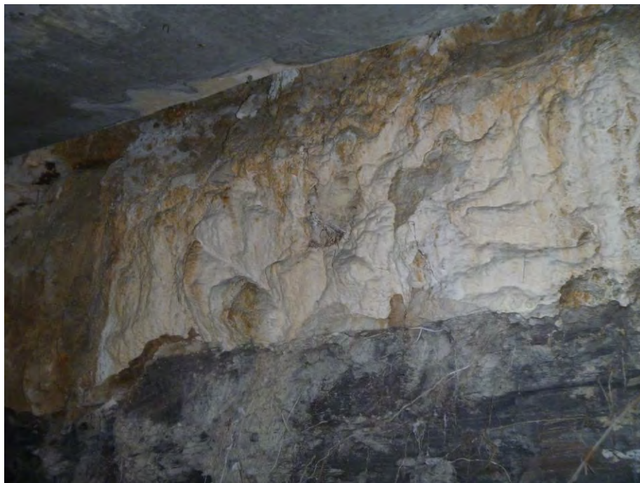
Photo 2 – Calcite staining (i.e. sign of groundwater seepage) on sandstone cutting in Car Park Level B4. Circled area in Photo 1.
