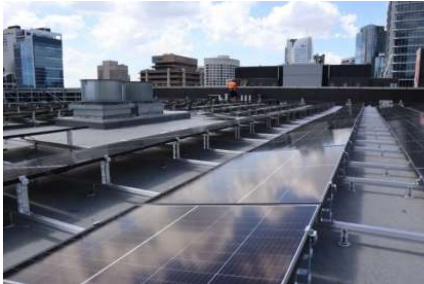
Figure 10 PV Solar on Roof
