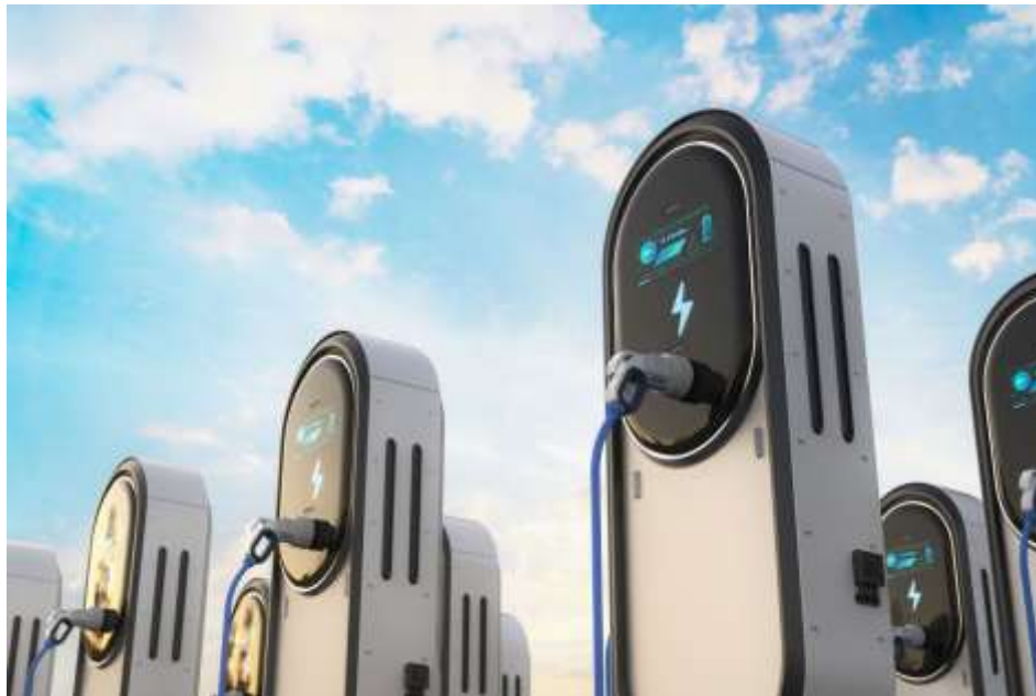
Figure 12 EV Charging Infrastructure
