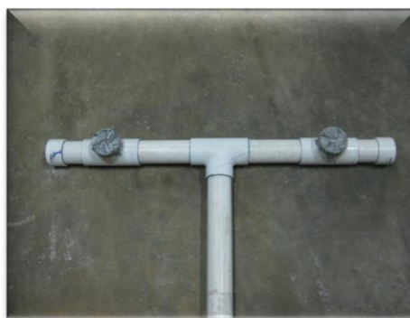
Figure 6. PVC Under Concrete Slab.
