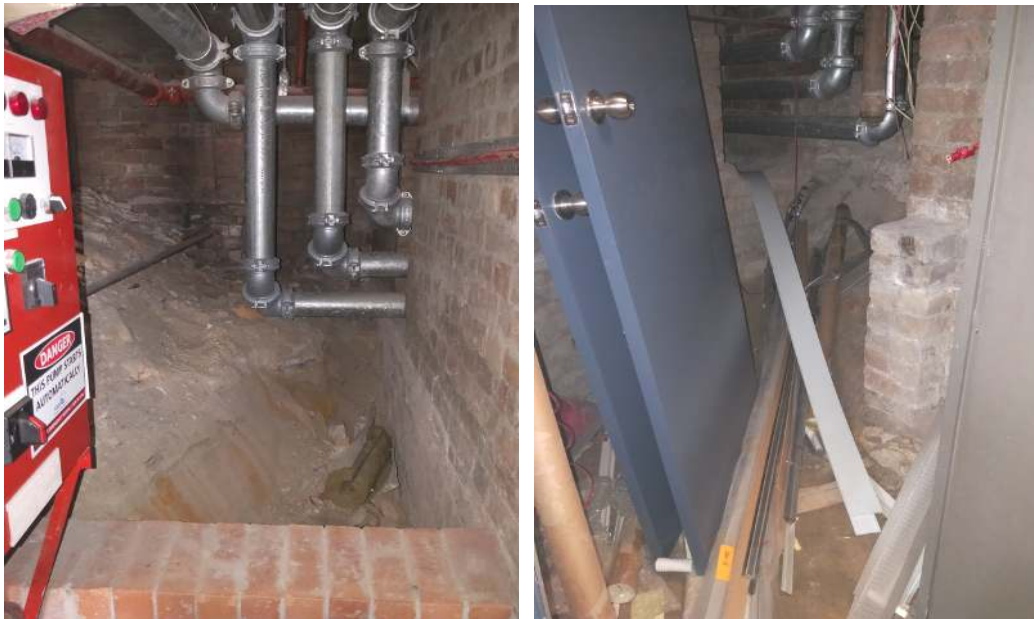
Photo 10 - Sandstone observed in the Pump room (L) and basement (R) of the Wilkinson House.
