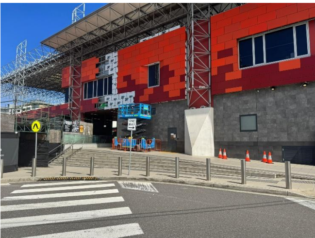
Newcastle Interchange at the corner of Station and Charles Streets, looking southeast
