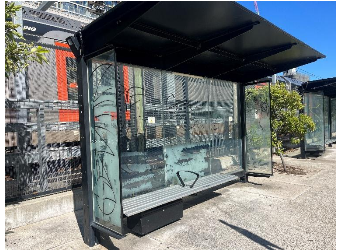
Graffiti and vandalism, Station Street
