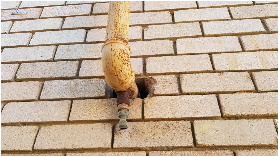
Photograph 3 Crevice in a building comprising potential and marginal microchiropteran bat roosting habitat
