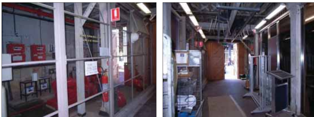
Figure 81: Plant room and entrance of Bay 2
