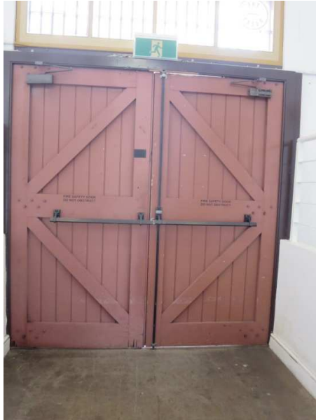
Level 2 Bay 5 Existing entry Door 5L2/XD1 Existing panic bolts to be replaced and new mounted at the compliant height.
