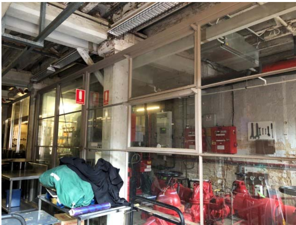
54 Pump room in Bay 2, ground floor level.
